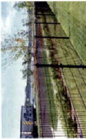
Sliding vehicular gate with automatic operator
